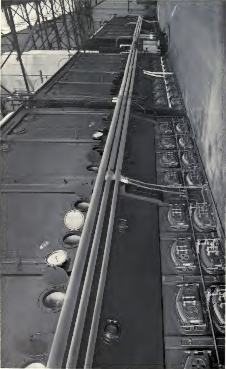
SOUTHERN CALIFORNIA EDISON CO., LONG BEACH, CAL. BABCOCK & WILCOX SUPERHEATERS INSTALLED IN 6200 HORSE POWER OF STIRLING BOILERS
